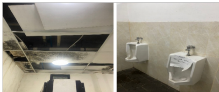
Figure 4. Toilet Condition (Source: Observation Results, Year 2026)
